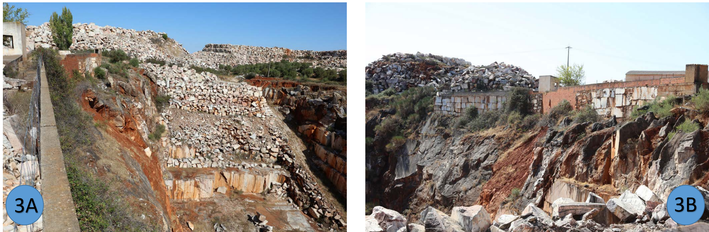
(3) Example of slope stability of the southwest slope in a quarry with suspended mining, which configures a situation like to that of the M255 road, with the "Dips" software. In truth, and luckily, situations like this are not the most common. (3A) View to the northeast; (3B) Southwest view; (3C) Planar sliding situation; (3D) Wedge sliding situation.
